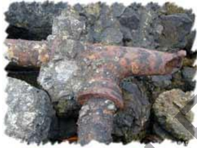
THESE PIPES ARE IN THE MIDDLE OF CHEMICAL CHANGES AS THEY RUST.
